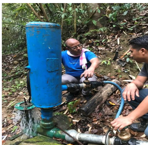
Figure 2. Ram Pump in operation in Nagaland. Image Courtesy – NEPeD, 2017
